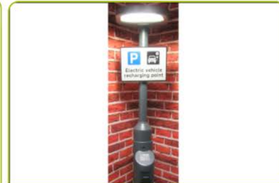
Opticharge - Lamp Column Charging Point
