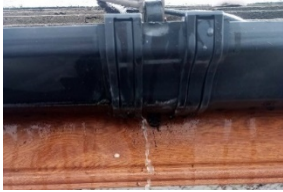
Figure 2 a: Leaking Gutter
