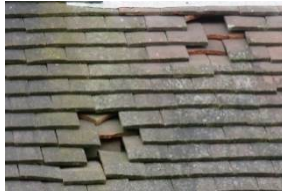
b: Damaged Roof
