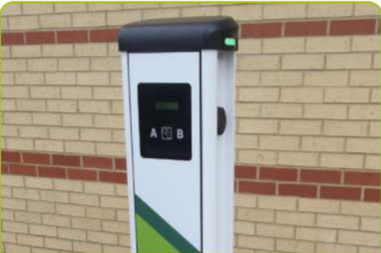
ePost - Charging Bollard
