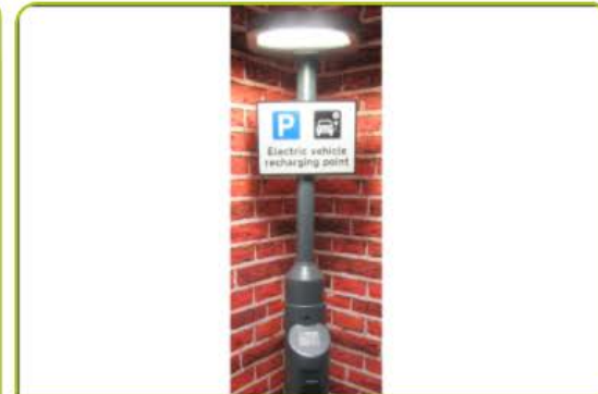
Opticharge - Lamp Column Charging Point
