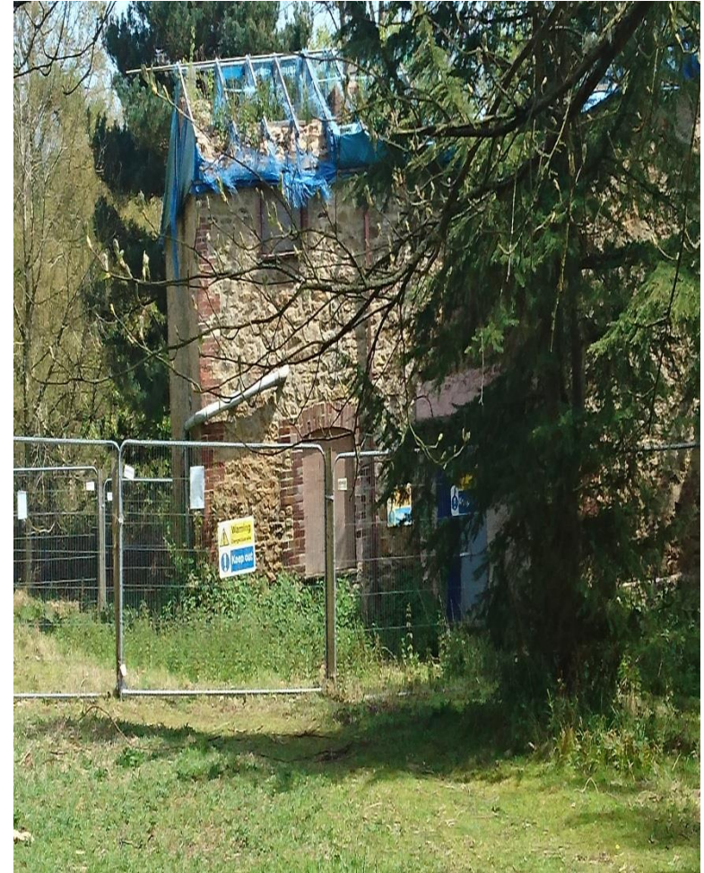
This picture shows the current state of the Farmhouse, which has an estimated restoration cost (per the Plan) of £63,000.
