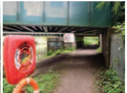
Poor quality riverside path (railway bridge over Thames)
